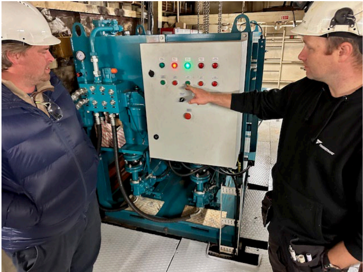
Figure 5: Photo of Bilge Support Arms HPU
